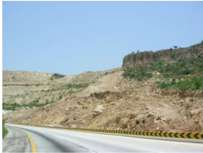
Figure 3.26 Slipped strata comprises large boulders (2-3m dia) in alluvial material
