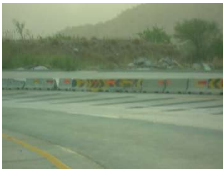
Figure 3.18 NJ Barrier on a sharp "s" curve showing damage by heavy vehicles
