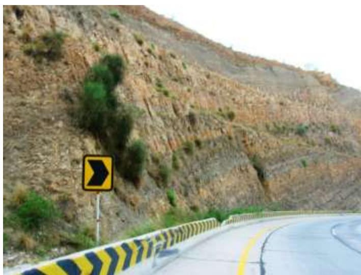
Figure 3.24 RCC Barrier showing damage by falling boulders
