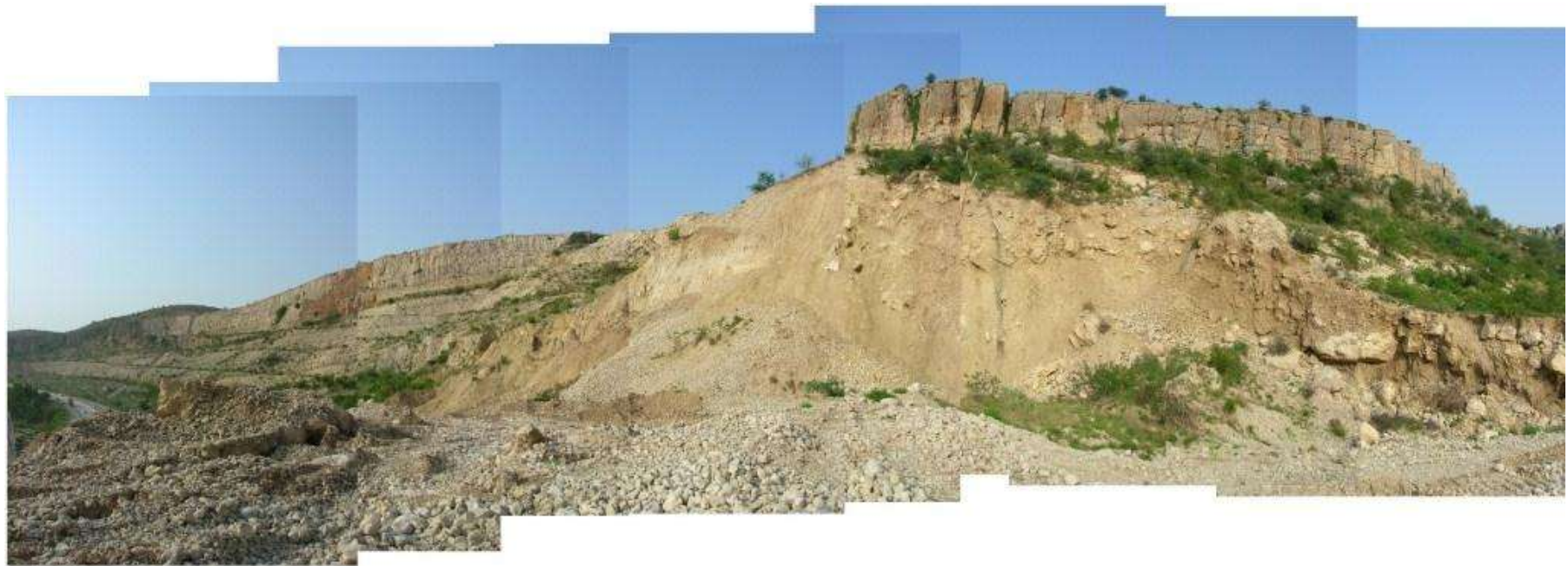
Figure 3.32 A panoramic view of the land slide near Simbal Motorway is visible on the extreme LHS
