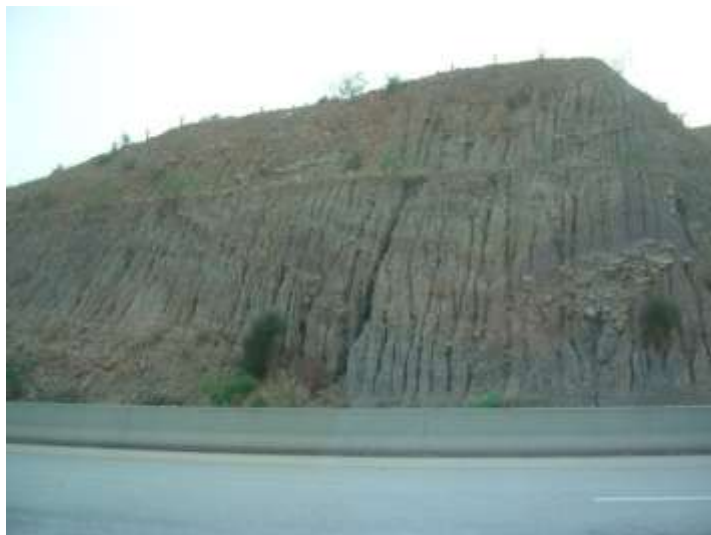
Figure 3.21 Erosion in weak soil along the alignment
