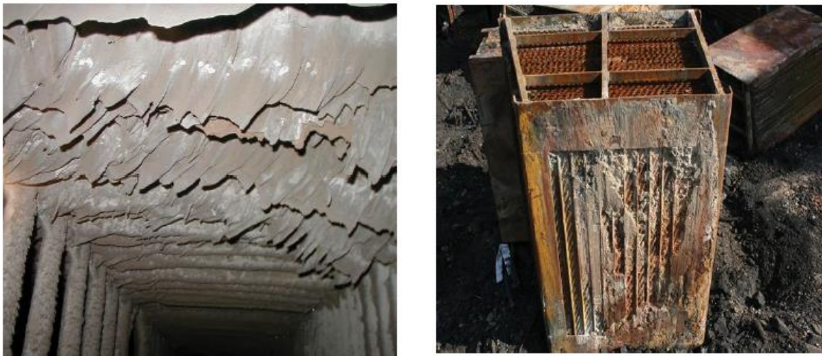
Figure 2.1: Ash slagging in the heat exchangers
