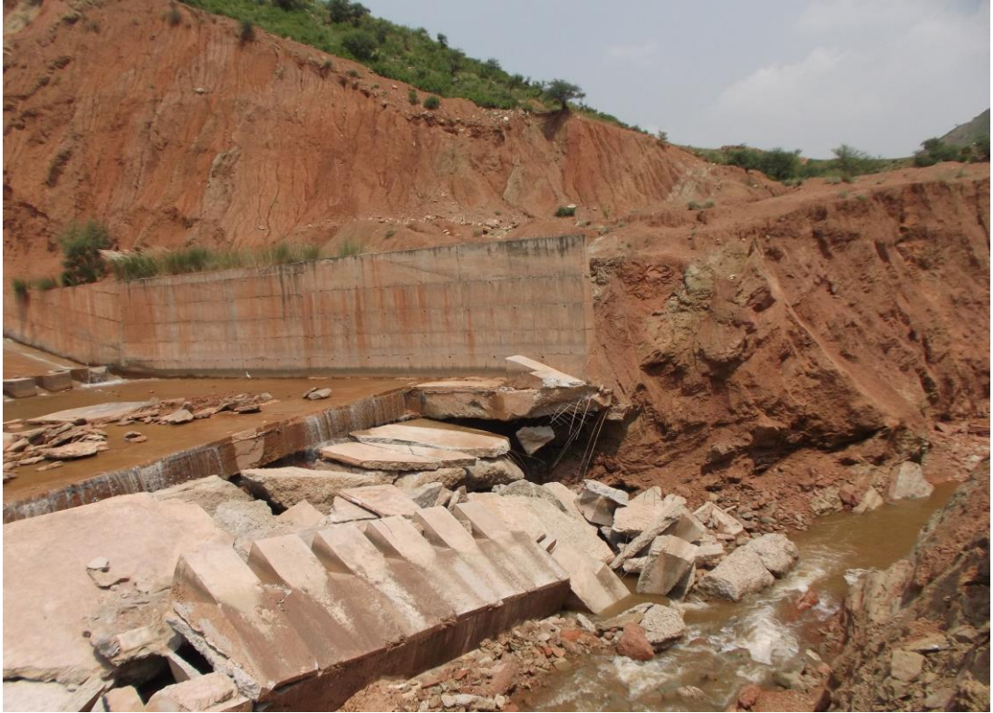
Figure 1.2 Broken stilling basin of Domeli Dam
