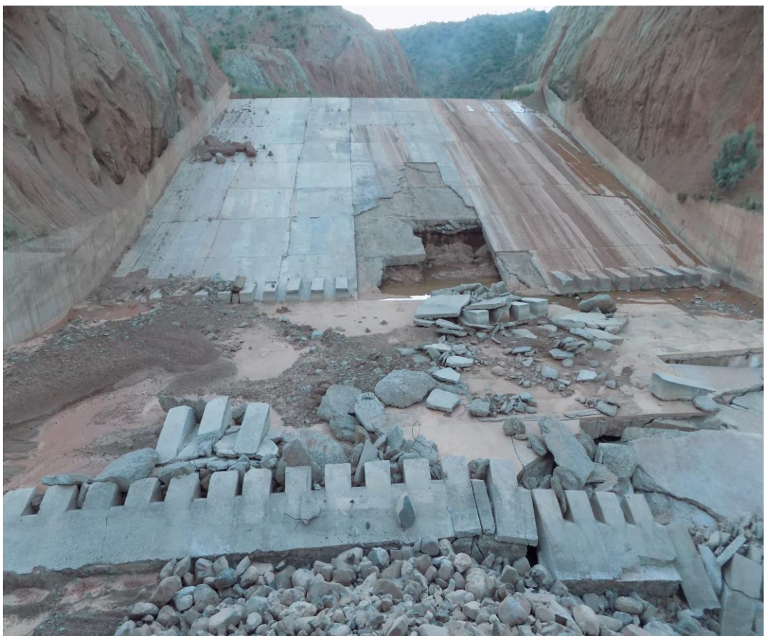
Figure 1.1 Broken stilling basin of Domeli Dam
